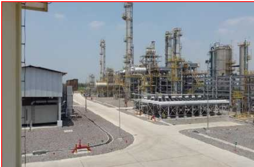
Gambar 08. Gas Turbine 4 x2,5 MW PT. Pertamina CPP Gundih.
